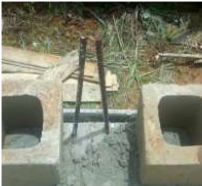
Plate V: Extension of 2Nos without bars from foundation for column extension due to lack of quality assurance.
