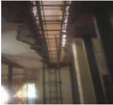
Plate II: Remedial works on ALIMS Building due to poor workmanship.
