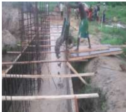
Plate IV: Casting of concrete into water filled formwork due to poor supervision.
