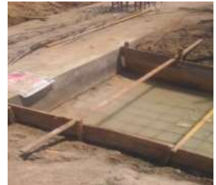
Plate VI: No provision of concrete groove at Joint.
