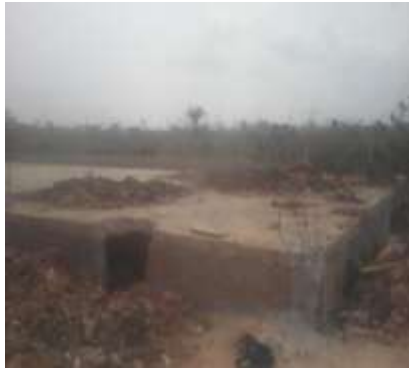
Plate I: Collapsed building site at Anambra state due to poor supervision.
