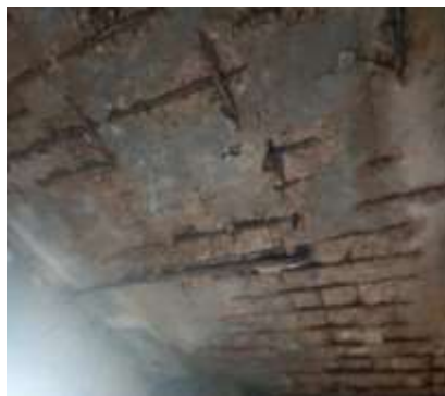
Plate VII: Rusted steel reinforcement bars in slab.
