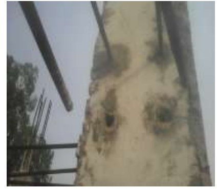
Plate III: Inserting of steel reinforcement bars into holes bored on column for beam.
