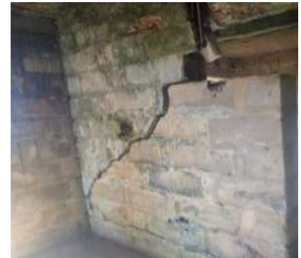
Plate IX: Cracked block wall with due to poor workmanship.
