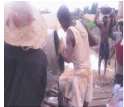
Plate XII: Mixing of concrete with dirty water due to lack of quality.
