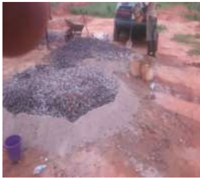
Plate X: Mixing of concrete on bare floor due to poor supervision.
